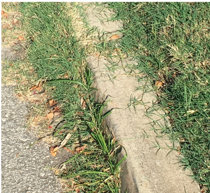
This curb is not properly maintained. Roots will weaken the structure and water will pond.
